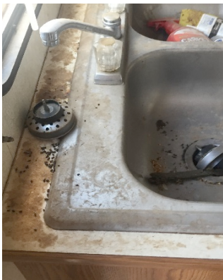
Figure 1. Rodent droppings along back of sink and in sink of a vacant trailer.
